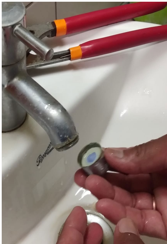
Water Aerator Installed in all
